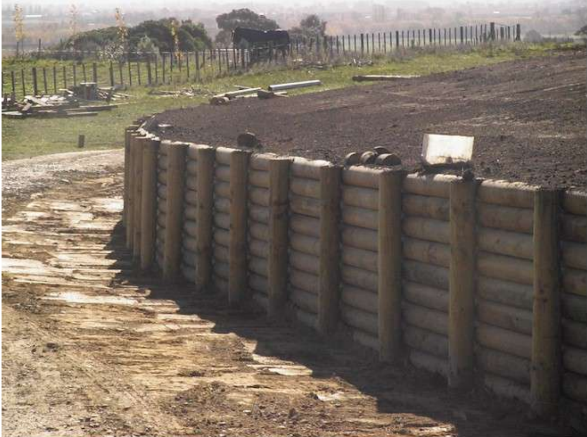
These piles were driven 3 meters into the ground with a deadman anchor system used to support the earth behind.
