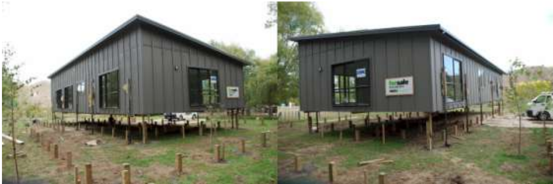
This $250,000 relocatable Titan home is in the process of being jacked down on site
