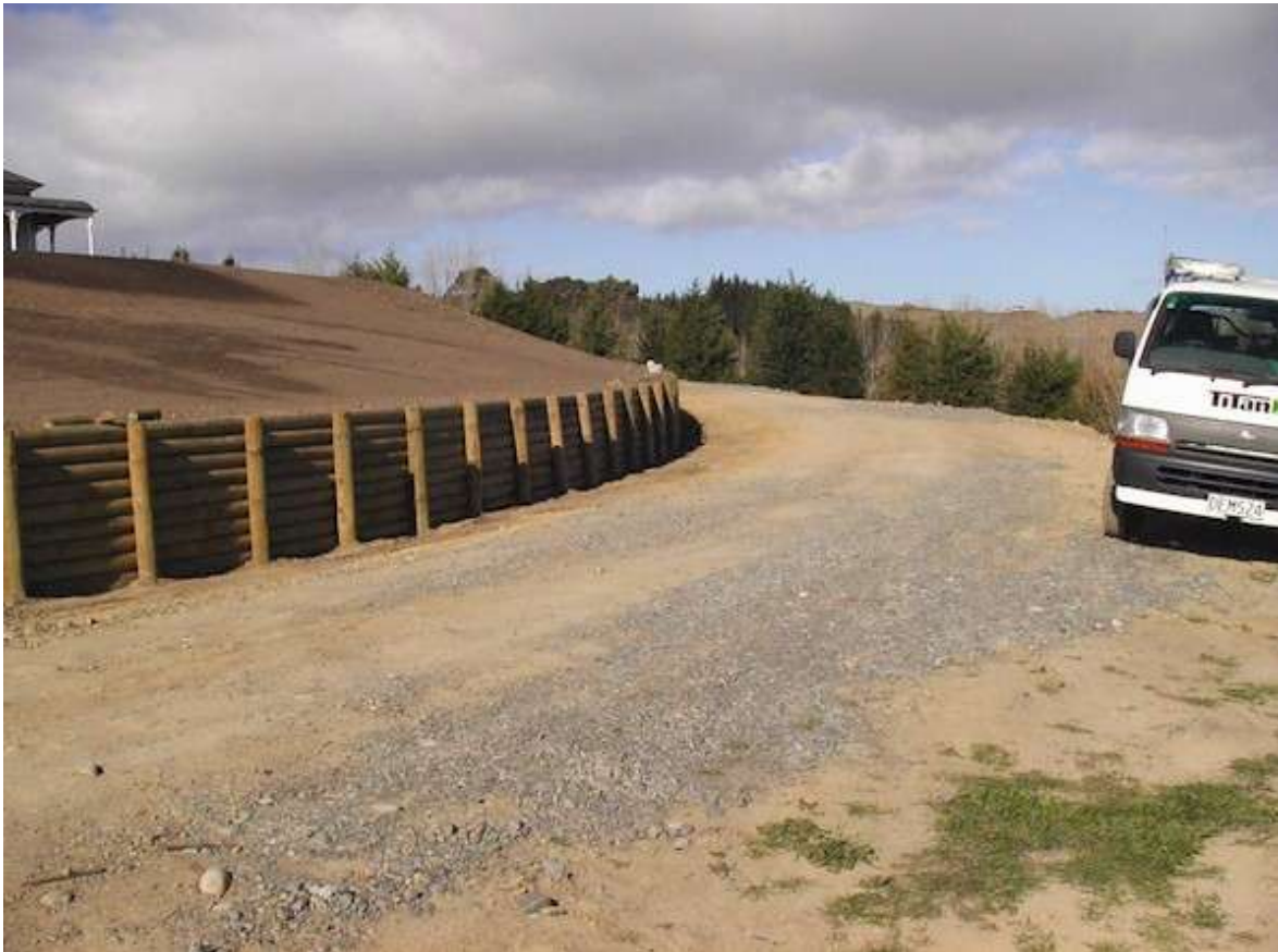
Some examples of retaining walls and landscaping that Titan Buildings have been involved in over the past 12 months
