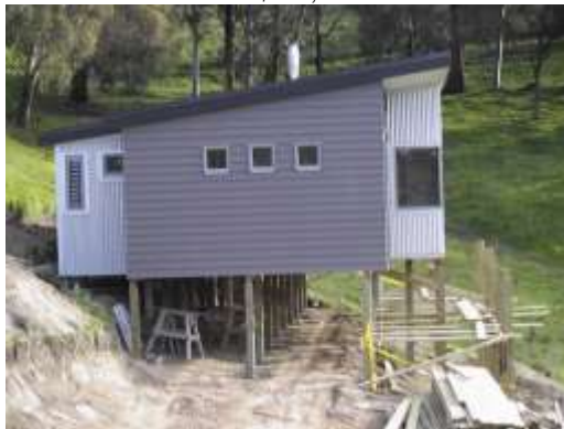
Extensive earthworks were required so that this relocatable home could be brought on to this sloping site
