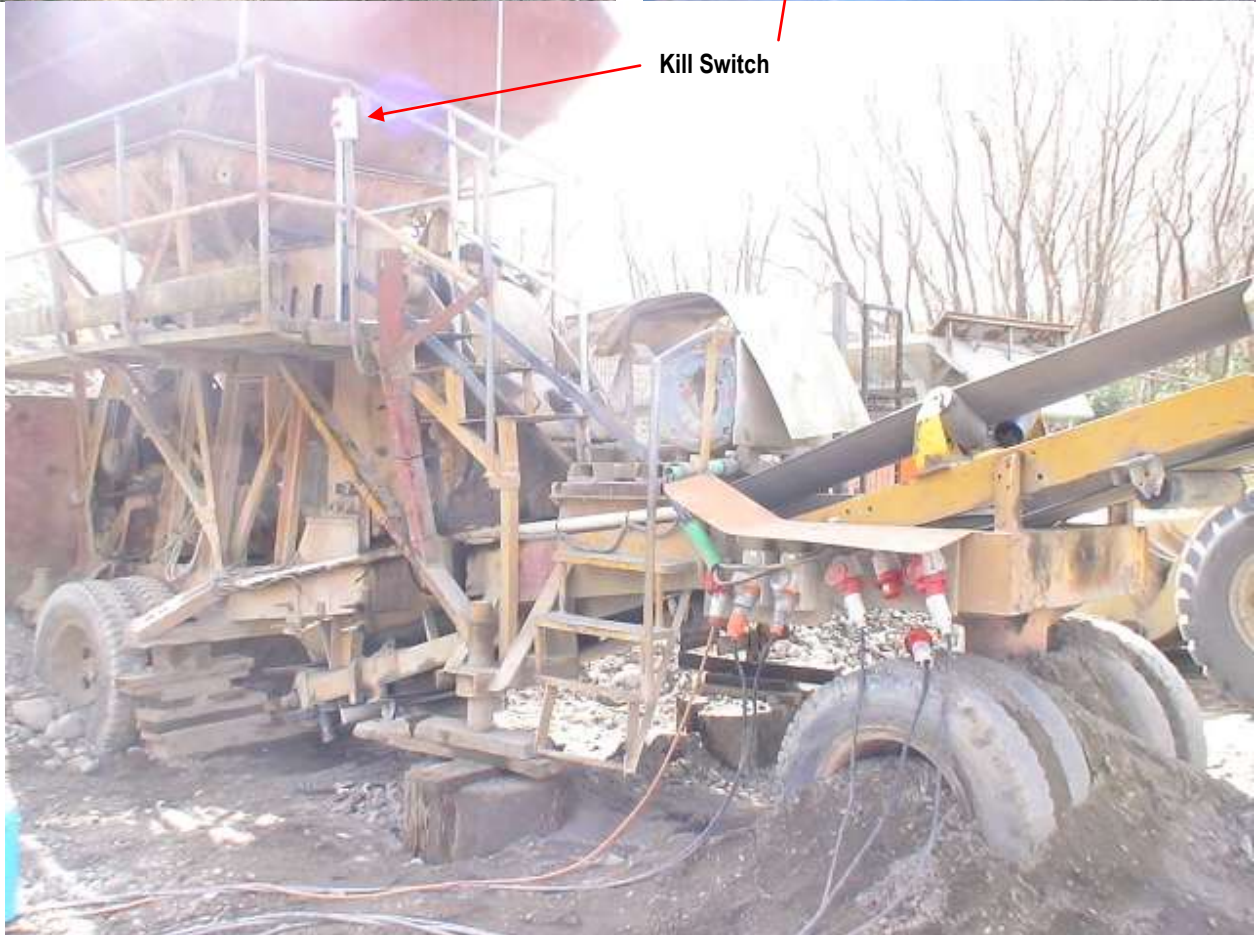
View showing the Crusher Operators vantage point and electrics
